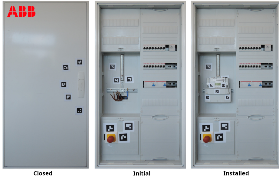
Fig. 6. The fuse box we use for our demonstration: On the left side the door of fuse box is closed. The fuse box’s initial state with opened door is depicted in the middle and the fuse box’s state of an installed electricity meter is shown on the right side
